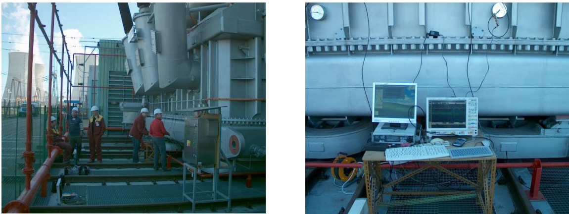
Figure 21 Measuring setup in nuclear power plant
