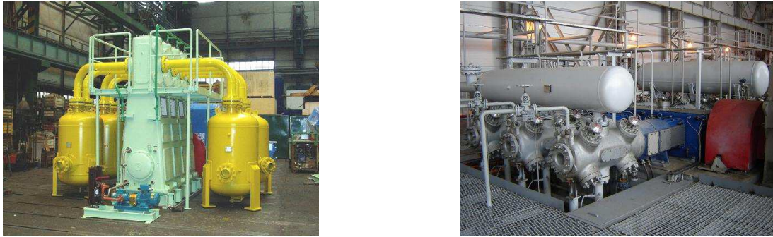
Fig. 1 – Reciprocating compressors operated in chemical industry facility
